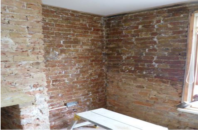
Dryshield applied to left hand wall and half-way down right hand wall.
