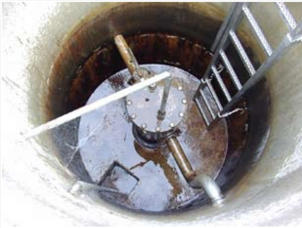
The leaking area
